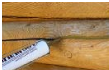
Fill checks and cracks.
